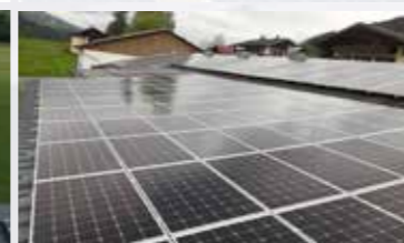
Neuwirth Pruggern, 100 kWp
